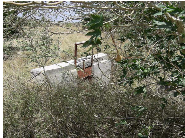
Canal intake at Hawaay. The canal needs rehabilitation
