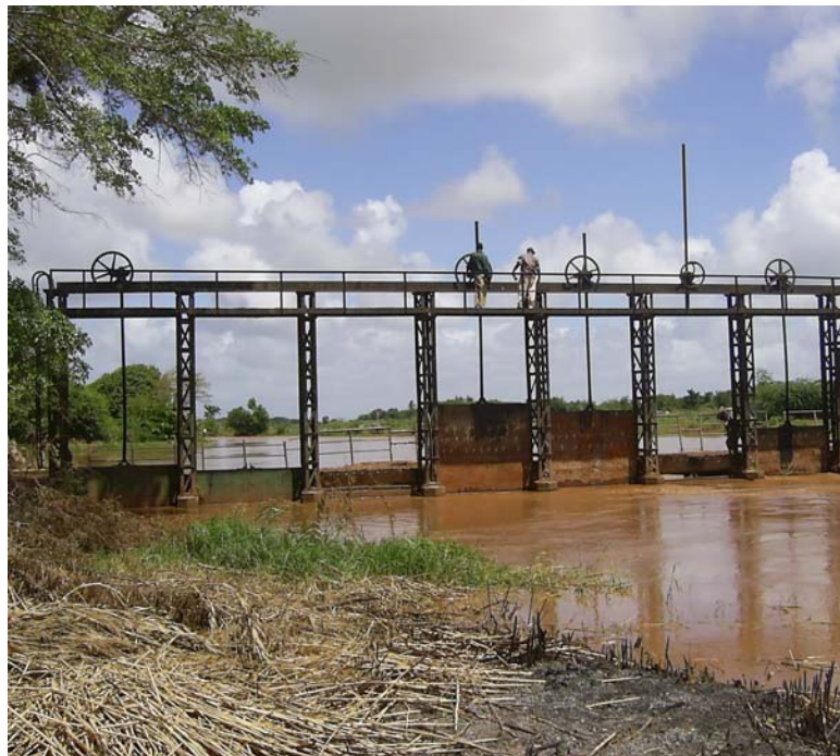
Qoryooley barrage before rehabilitation. All gates were corroded and sunk in the mud.
