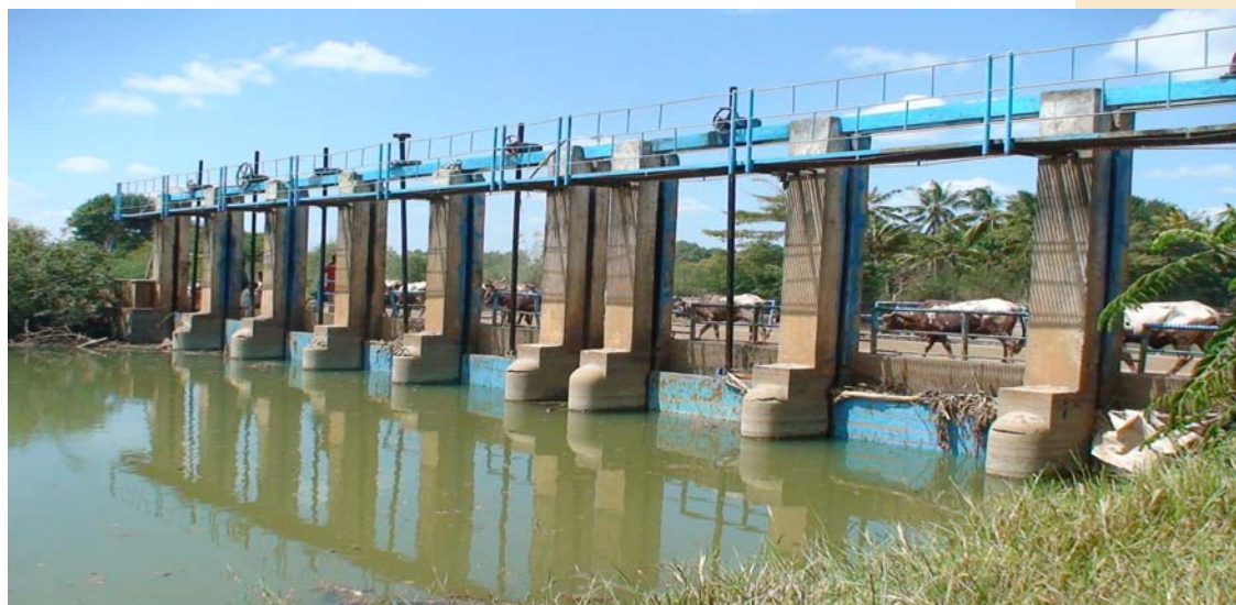
Falkeerow barrage after rehabilitation by SWALIM in 2009. New lifting gears were installed for operation of the gates. Some of the gates were rehabilitated and all barrage structures painted.
