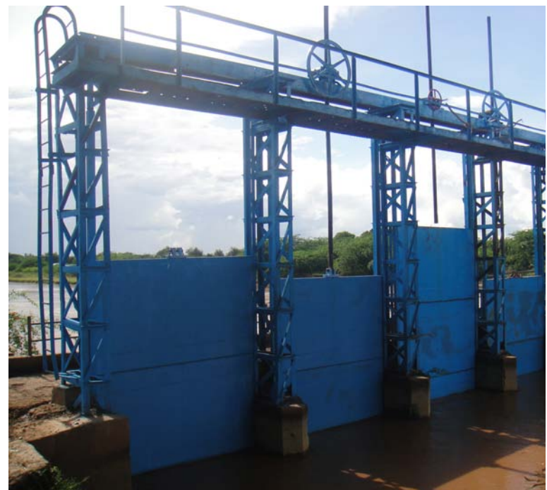
Qoryooley barrage after rehabilitation by SWALIM in 2009. All nine gates were replaced, old gears were serviced and three lifting gears were installed to the barrage.
