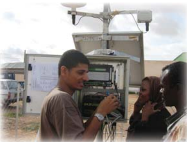
Installation of an automatic weather station at the PSAWEN compound in Garowe, Puntland
