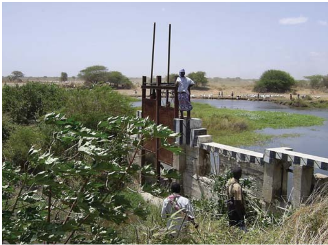
Haway Barrage – note that no water is flowing through the gates, which was the original water course. The river bed is now full of vegetation. The water in the background is the new river course, which bypasses the barrage.
